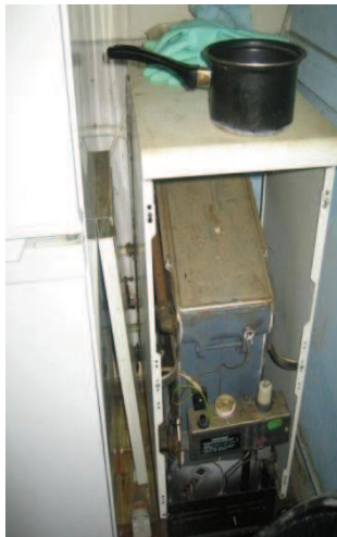
Damaged boiler with front panel missing
