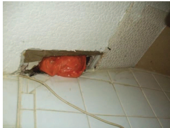
Hole in kitchen ceiling stuffed with plastic bag
