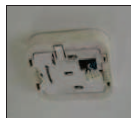
Disabled smoke alarm with the cover removed
