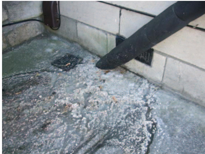
Blocked front drain
