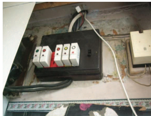
Fuse board, dated and no earthing
